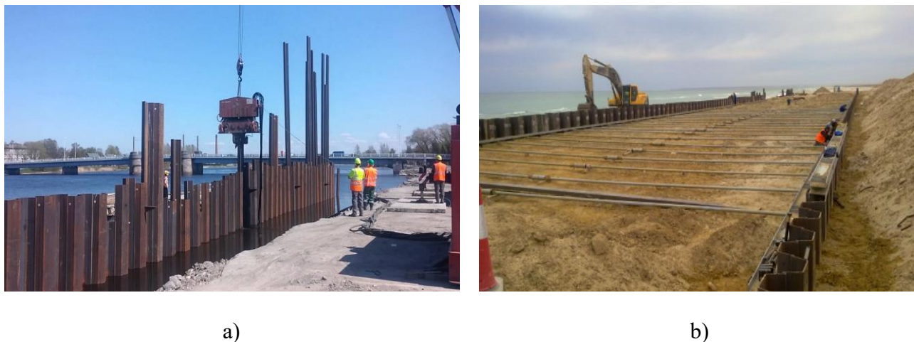
Figure 2 – Installation of tongue-and-groove piles on the left bank of the Moskva River embankment in Krasnogorsk, Russia (a). Krasnogorsk (Russia) (a) https://arcticgs.ru/stati/stroitelstvo-prichalov and on the shoreline of the Kazakhstan Offshore Industries production base in Akshukir (Kazakhstan) (b) https://www.instagram.com/p/CU7Af8XILkT/?img_index=1
